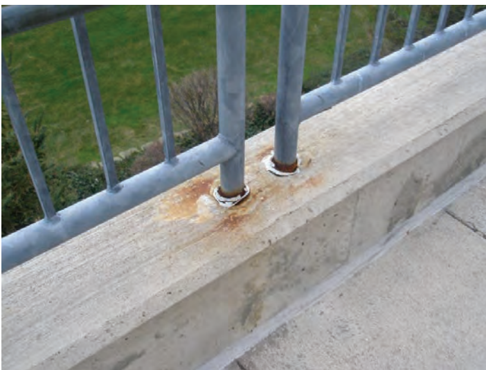
C2 - Typical failed sealant at guardrail post
