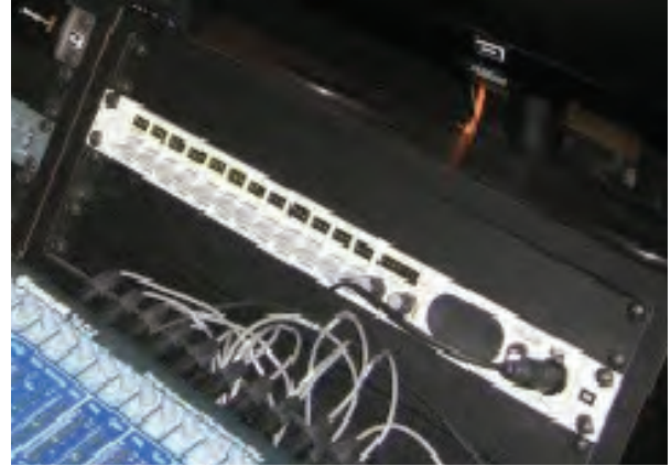
T3 - Intercom Panels
