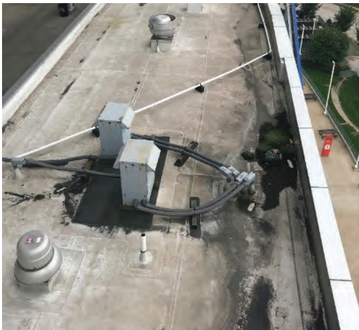
E3 - Upper concourse roof top transformers over concessions
