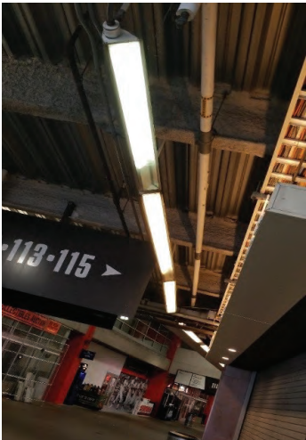
E6 - Main Concourse linear fixture
