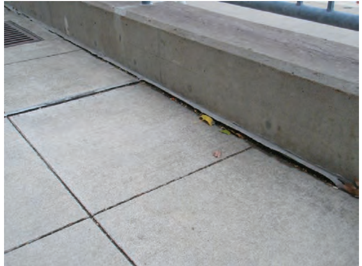
C3 - Typical failed sealant on plaza
