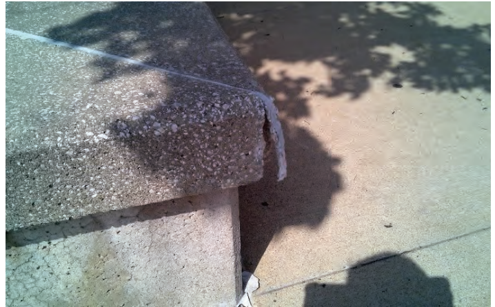
L6 - Planter bed precast concrete coping - poor condition
