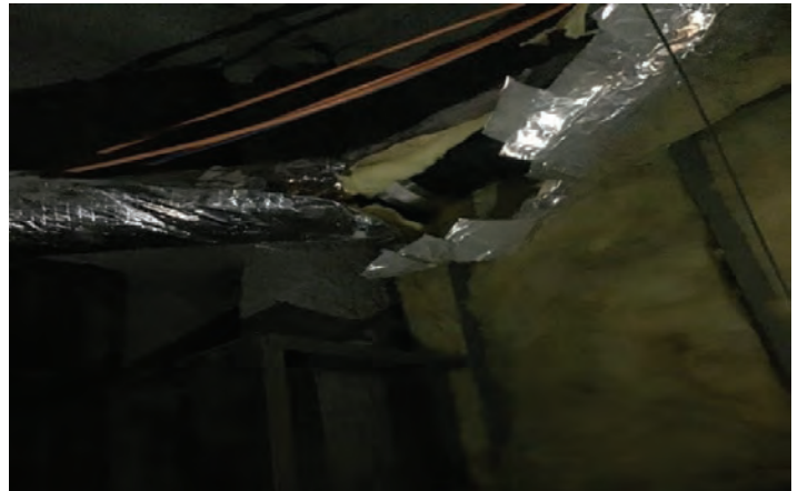
p2 - Unsecured Insulation in Suite Level Ceilings
