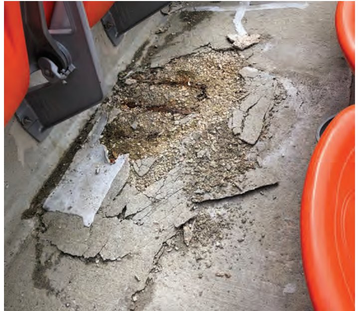
S1 - Typical Spalled Concrete
