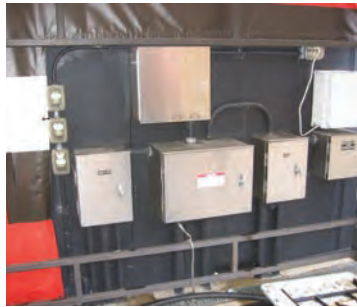
T1 - Stadium Interface panels
