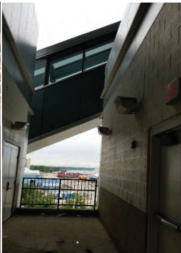
E7 - Typical wall mounted HID Fixture
