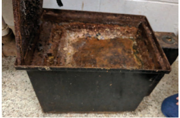
P6 - Rotted Grease Trap
