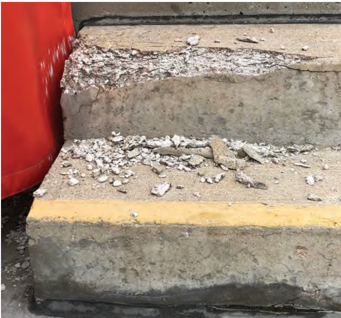
S4 - Typical Deteriorated Aisle Step
