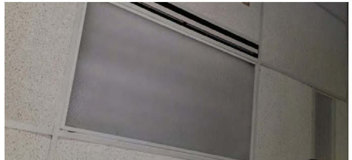
E13 - Typical troffer type fluorescent in "back-of-house" location
