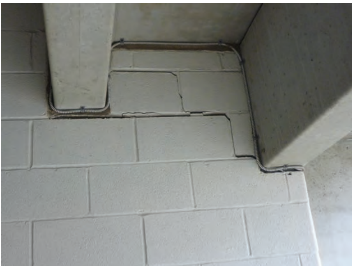
S5 - Typical Masonry Cracking at Vomitory Wall
