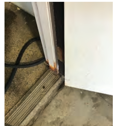
A4 - Typical hollow metal door rusting at base
