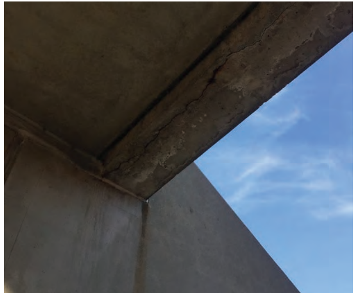
S2 - Typical Cracked Concrete
