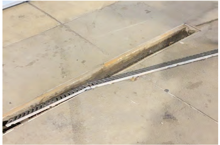
P3 - Unsecured trench drain gate
