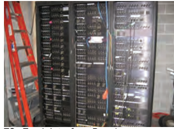
T2 - Truck Interface Panels
