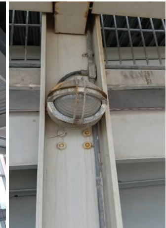
E5 - Typical interior ramp fixture
