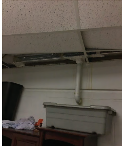
A13 - Water damage at finish ceiling
