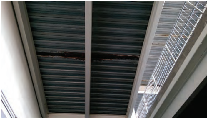
S8 - Typical Corroded Metal Floor Deck at Ramps
