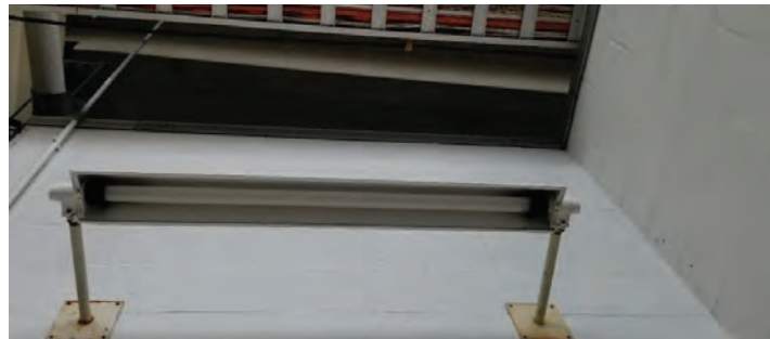
E9 - Linear fluorescent fixture in concourse
