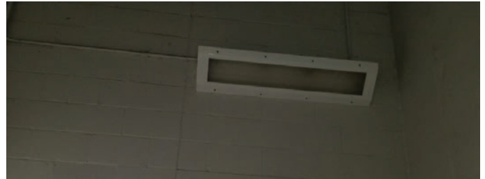
E11 - Typical toilet room corner mounted fluorescent fixture
