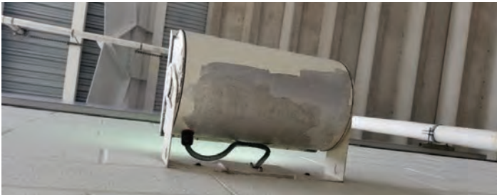
E8 - Typical wall mounted HID fixture showing corrosion
