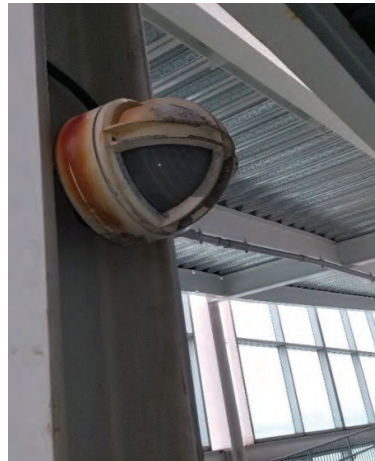
E4 - Typical interior ramp fixture
