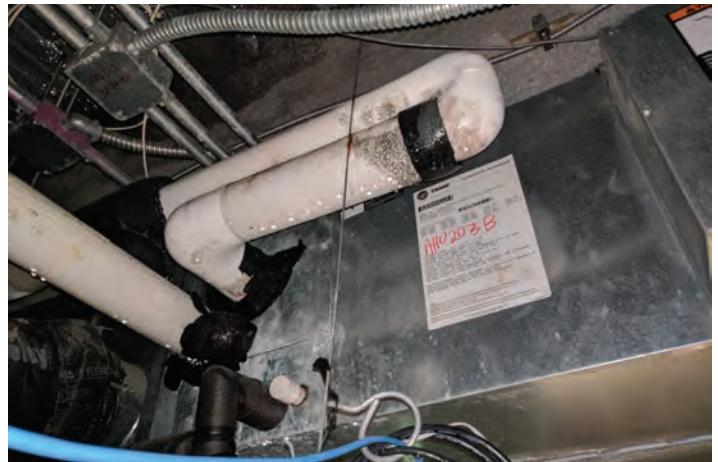
M1 - Water Saturated Insulation; FCU Chilled Water Piping
