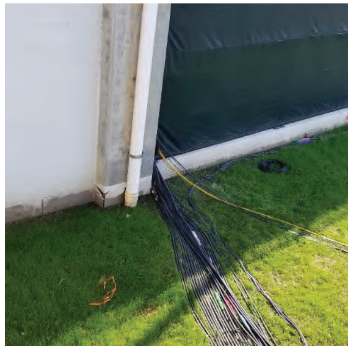
E16 - Temporary power cables entering service area
