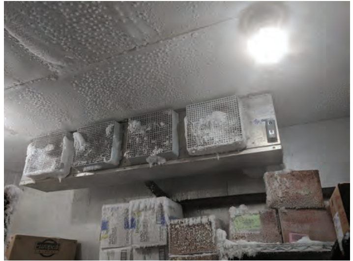
M6 - Ice Build-up on Evaporator and Freezer Contents
