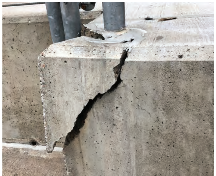
S3 - Typical Concrete Damage at Guard Rail Post
