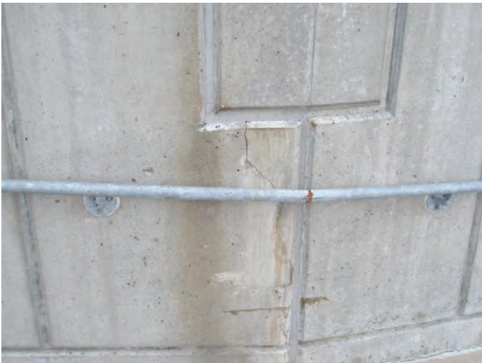
C1 - Typical Structural crack in retaining wall
