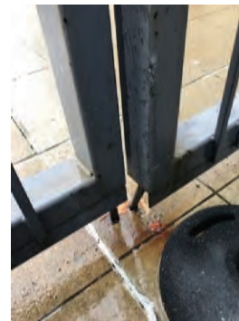
A5 - Typical security gate hardware (damaged cane bolt)
