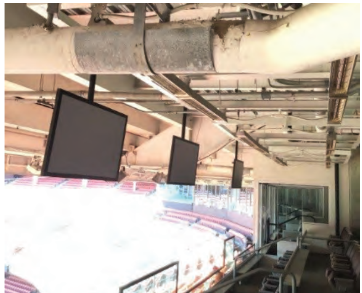
P4 - Disintegrating Storm Insulation
