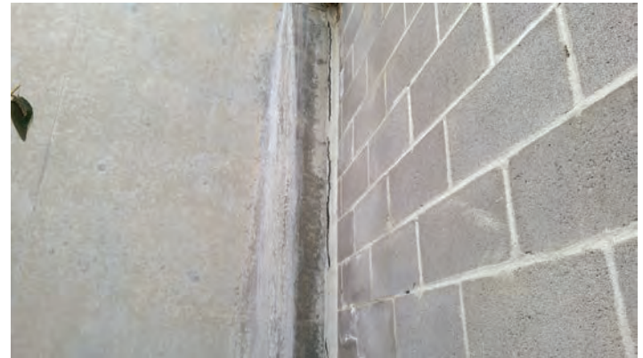
S6 - Typical Failed Backer Rod and Sealant Joint
