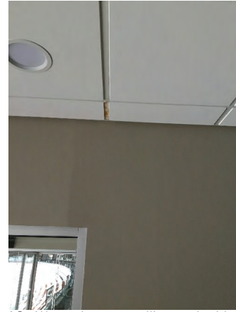
A8 - Water damage ceiling and grid
