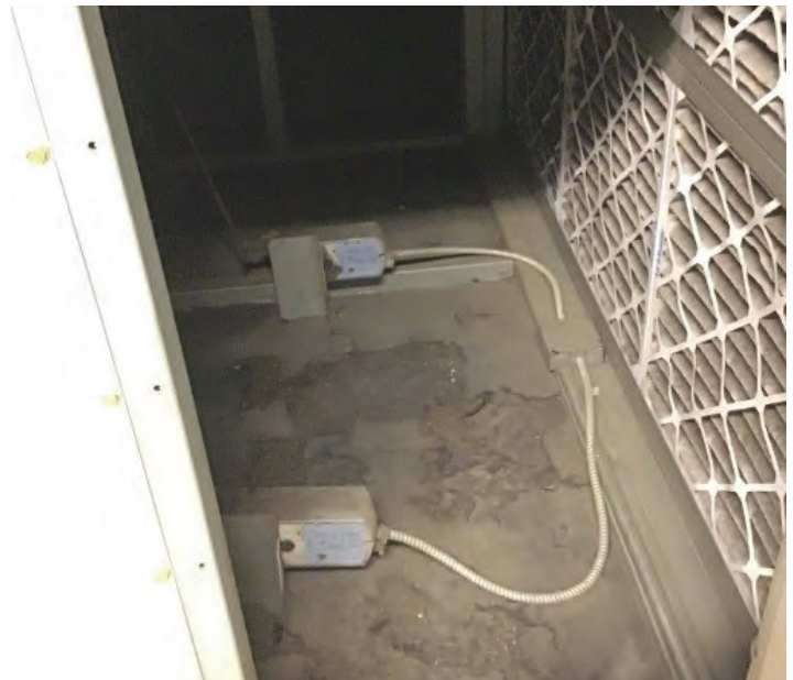
M2 - AHU Deteriorating Internal Lining
