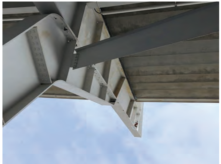
S9 - Typical Surface Corrosion on Structural Framing Member
